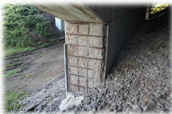
Delaminated Concrete Removed from Pier
