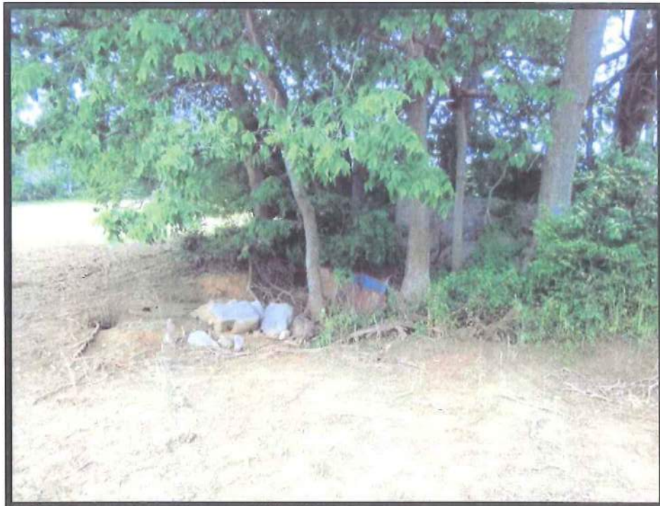
Attachment I: View of Sinkhole #2, Looking West-Northwest.
