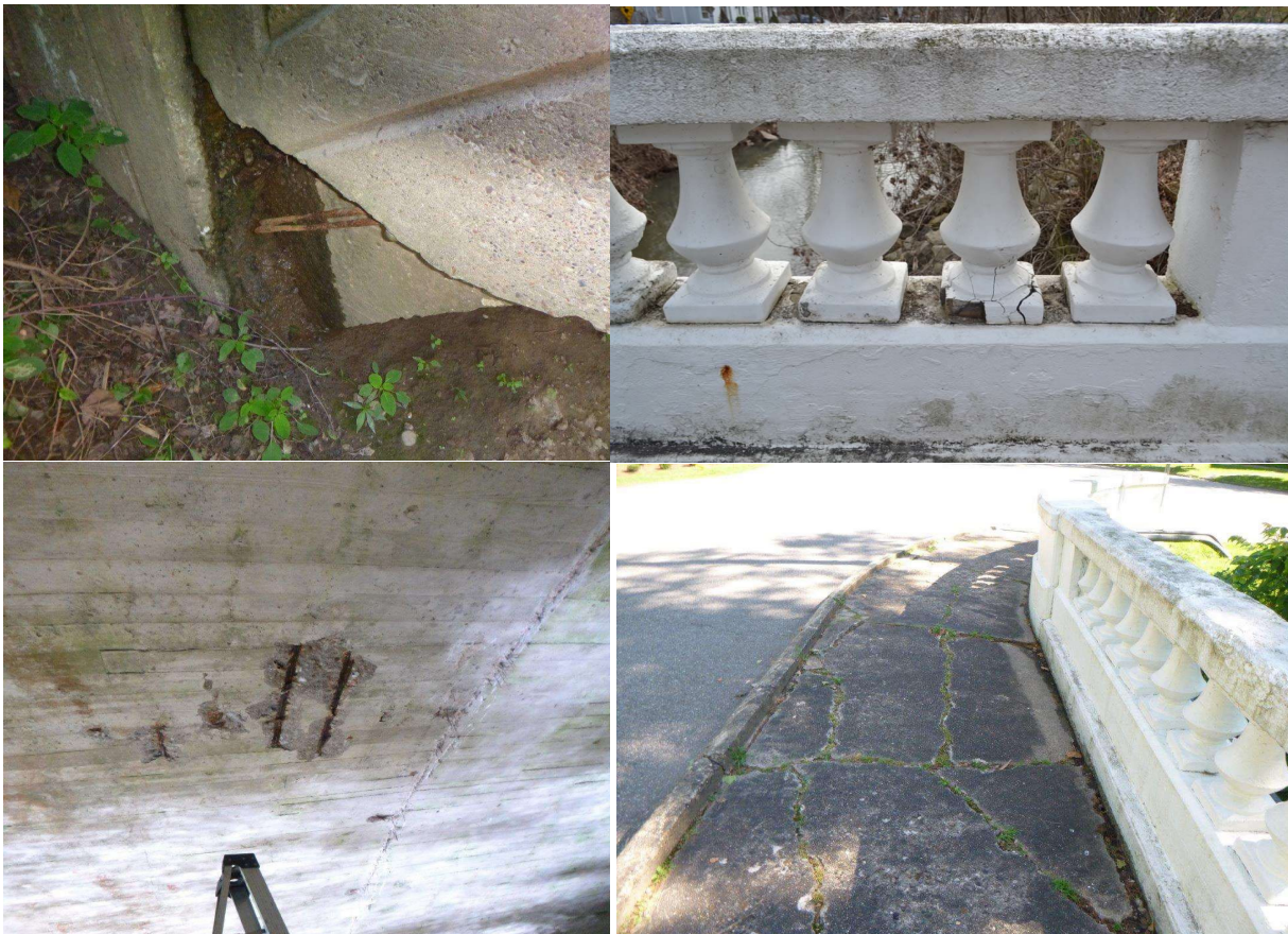
Figure 1. Photographs of the 12 th Street Bridge with varying degrees of deterioration.
