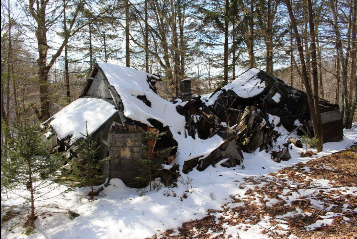
Photo 1. Roger Pennington Homestead showing southeast (front) and northeast (side) façades of collapsed dwelling, facing west.
