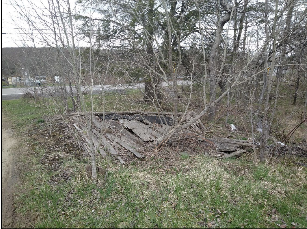
Figure 23: View facing west showing foundation and structural remains in the vicinity of the proposed US 219 interchange at Thomas
