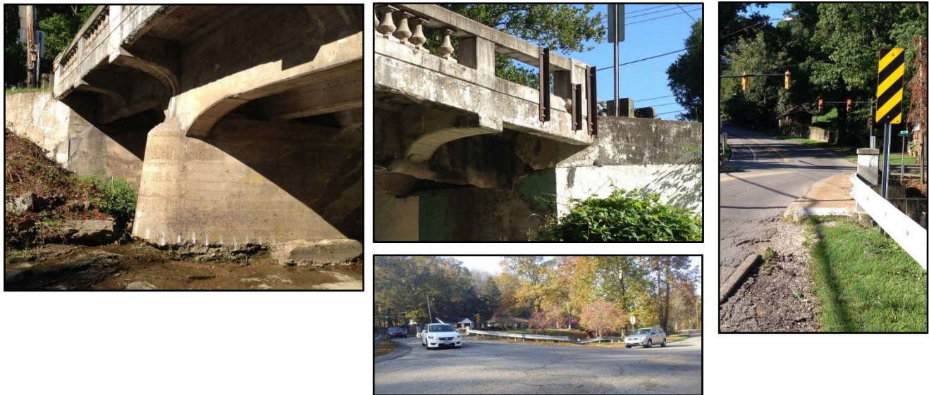
Figure 1. Photographs of the 5 th Street Bridge. Left: View of deteriorating pier. Middle Top: View of missing balusters and repairs. Middle Bottom: View toward the narrow bridge from North Boulevard. Right: View
