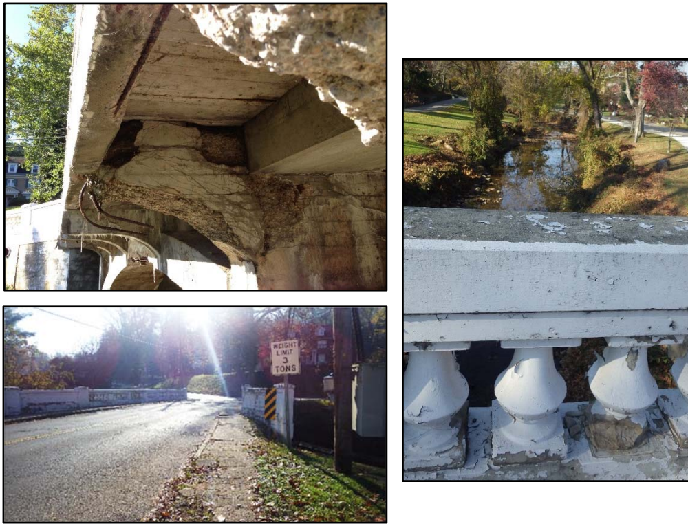
Figure 2. Photographs of the 8 th Street Bridge. Left Top: View of deterioration under the bridge. Left Bottom: View across the bridge facing south. Right: View of balusters.
