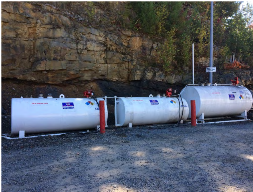
Photograph 12: View facing southwest showing the three ASTs located at the Aspen Corporation property.
