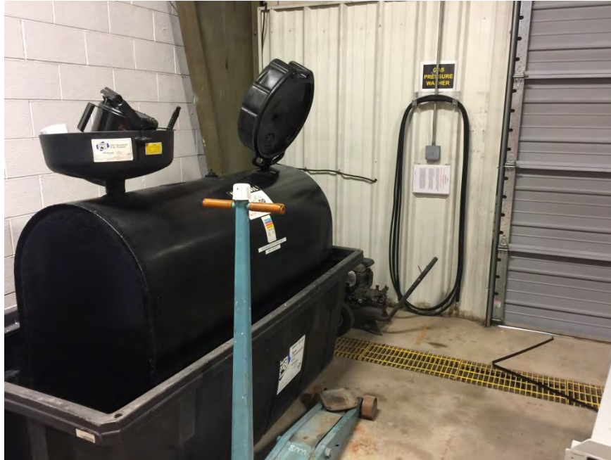
Photograph 19: View of the interior of the Heiner's garage showing AST containing used oil.
