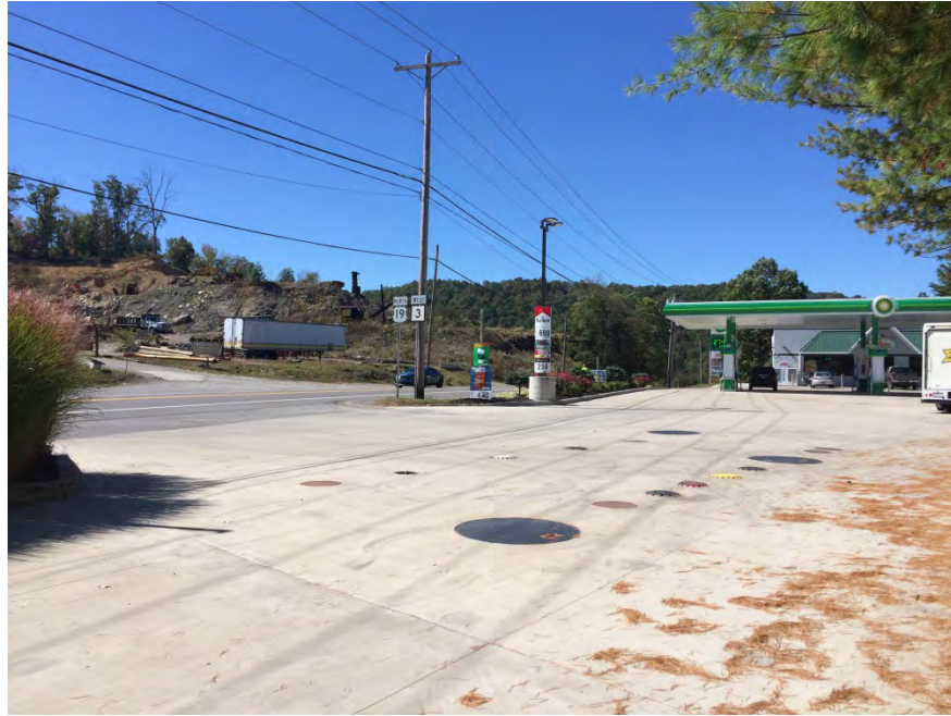
Photograph 13: View facing west showing USTs located at the BP Little General Store.
