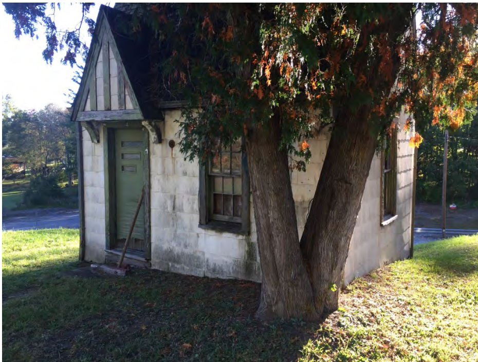
Photograph 10: View of small outbuilding located at the Sherry's Dinner property confirmed to have asbestos containing building materials.
