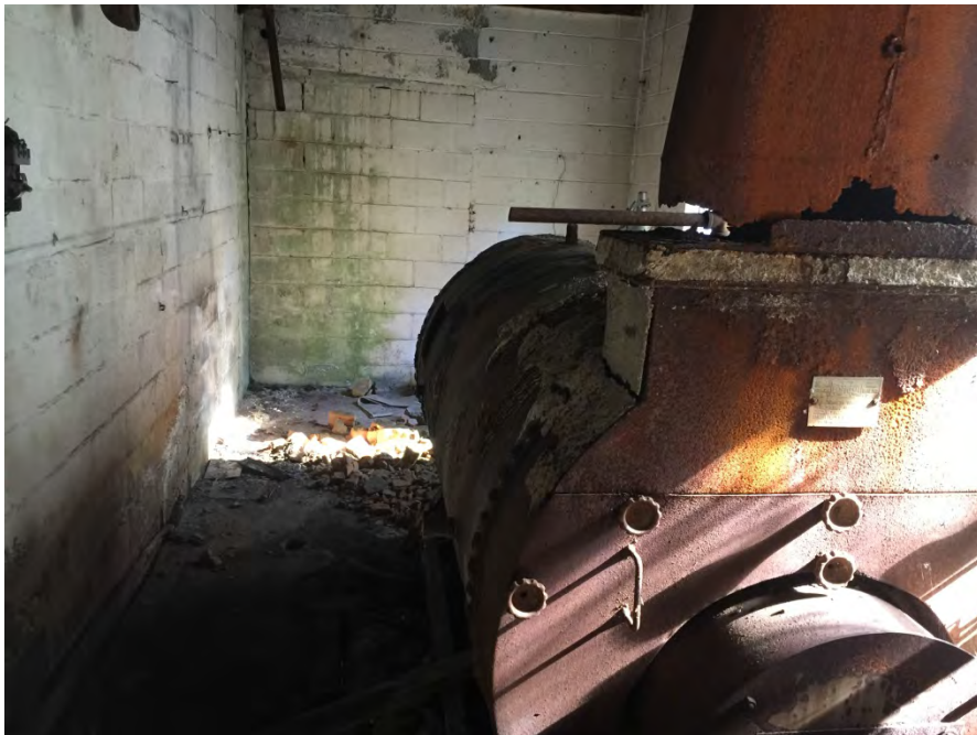
Photograph 24: View of the interior of the Peerless Packaging building showing burner/incinerator located on the southwestern portion of the building.
