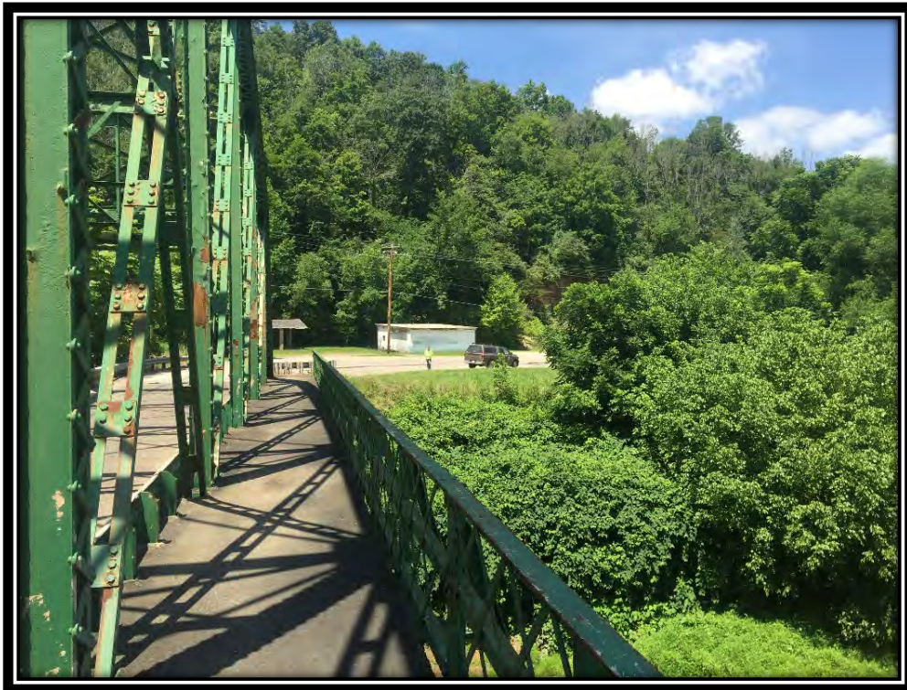
Photograph 4: View looking west across pedestrian crossing of bridge (former car wash in background).
