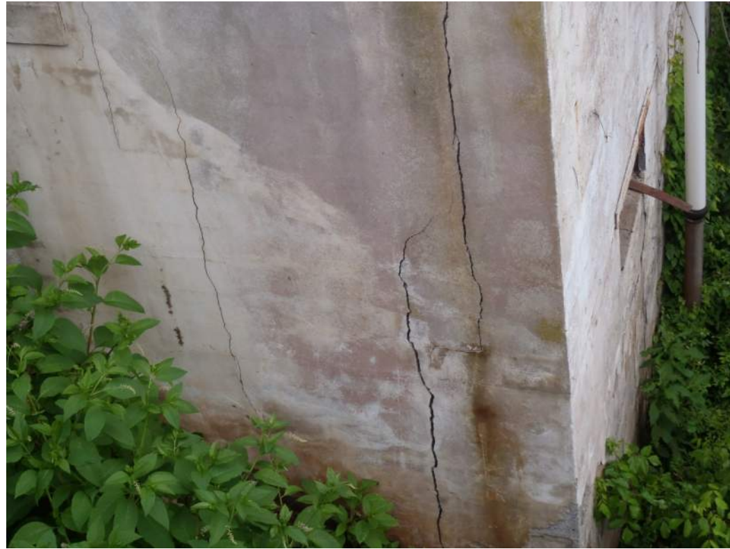
Photo 33: Large cracks in the foundation of the Richard's Tractor Sales building.
