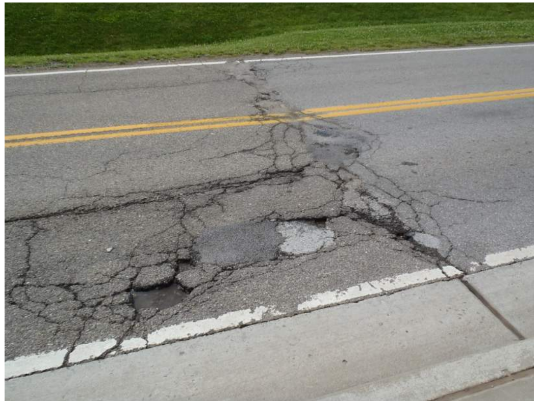
Photo 26: Section of Williams Drive detour route with poor asphalt condition.
