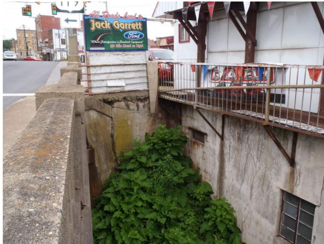
Photo 34: Foundation of Richard's Tractor Sales in contact with Abutment 1 of Ruby Bradley Bridge.
