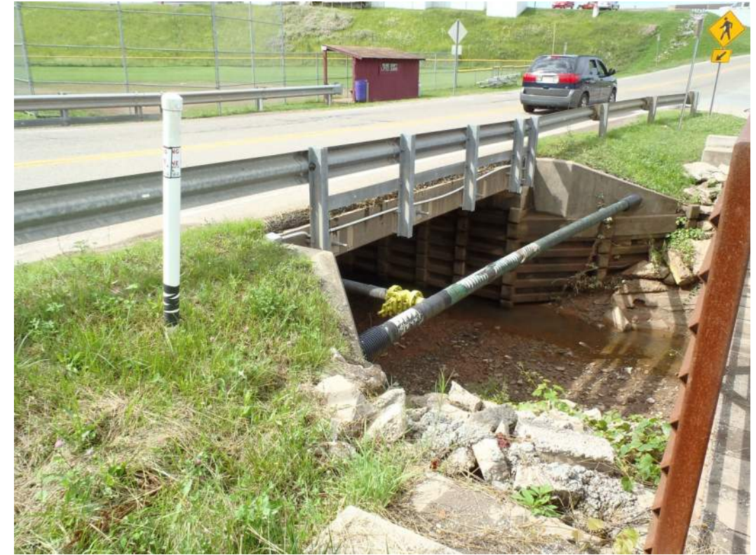
Photo 27: Bridge and aerial gas line crossing Goff Run along the Williams Drive detour route.
