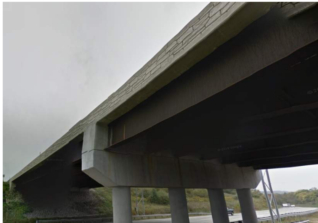
Photo 46: View of concrete stamping on the deck barrier of Three Springs Bridge.
