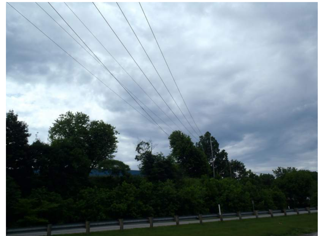
Photo 20: Overhead lines within the proposed alignment of the Williams Extension, Alternative 3.
