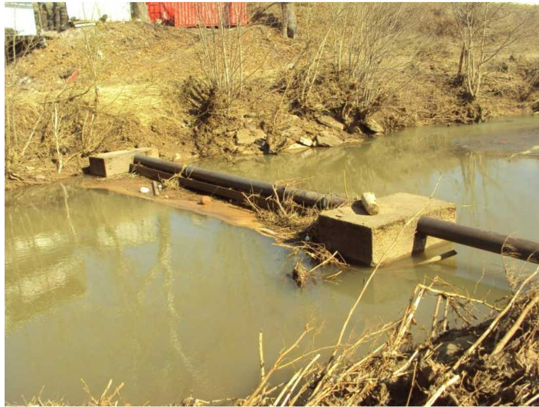
Photo 17: Abandoned aerial sewer crossing paralleling the downstream side of the existing bridge.
