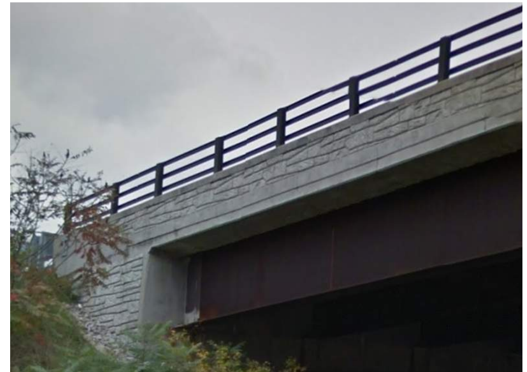
Photo 47: View of concrete stamping on the deck barrier and wingwall of Three Springs Bridge.
