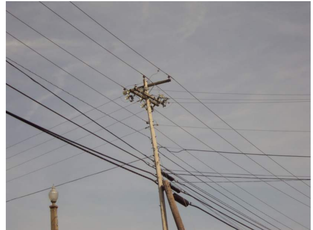
Photo 15: Overhead utility lines which parallel the upstream side of the existing bridge.
