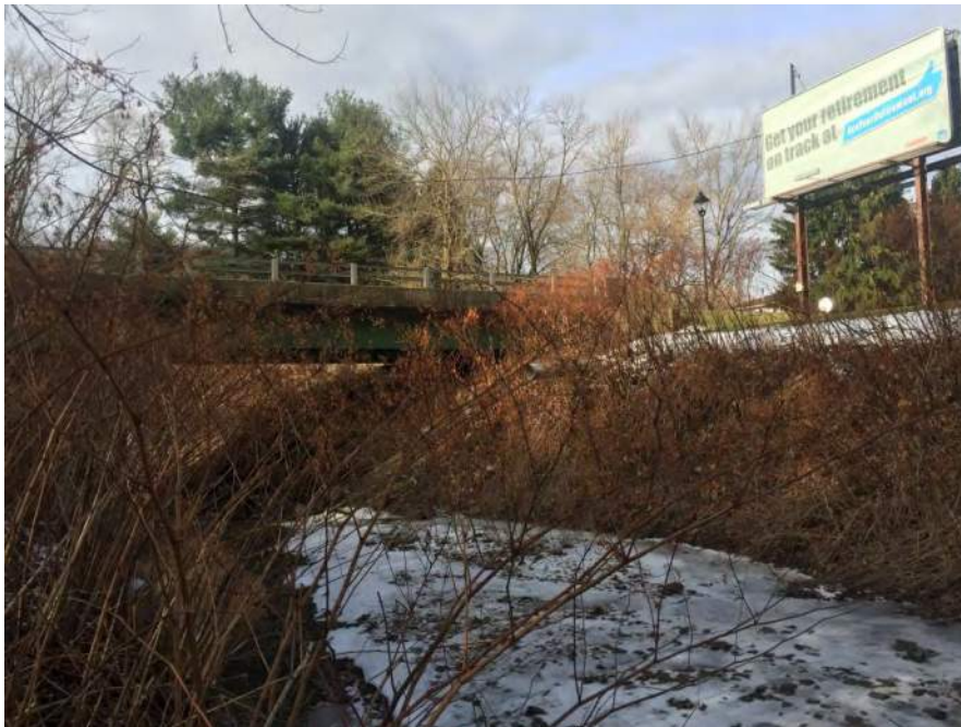
Photograph 2: View facing north showing the bridge that carries North Chester Street over Hardin Run.
