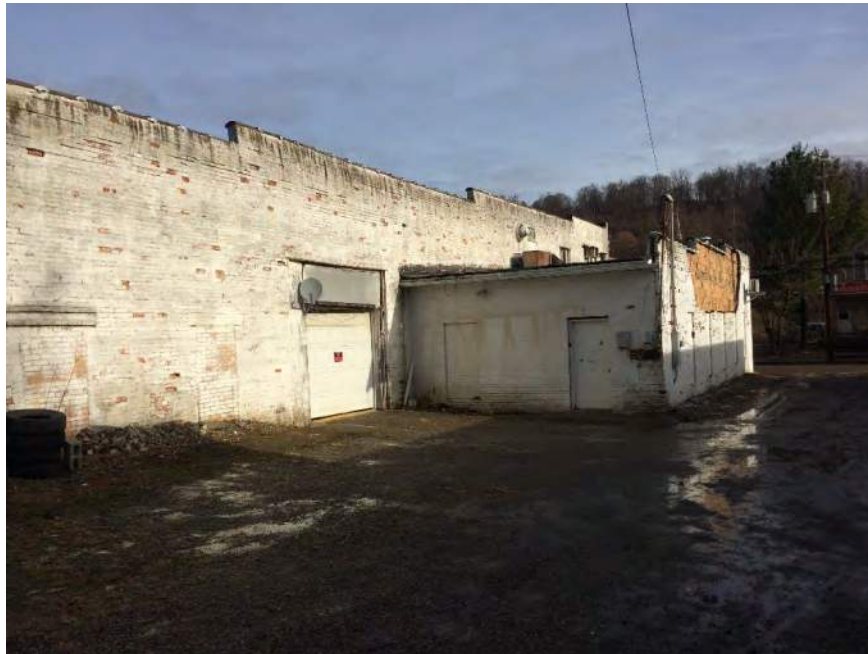
Photograph 18: Rear of building identified as Former Dry Cleaner looking northwest with South Chester Street in background.
