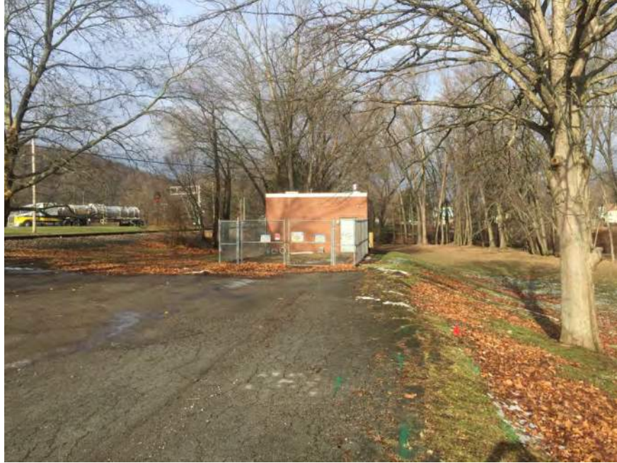
Photograph 5: View facing north showing municipal sewer vac station located in the New Cumberland City Park.
