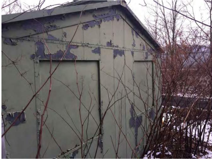
Photograph 5: Side of Columbia Gas Transmission Station showing flaking/peeling of potential Lead Based Paint.
