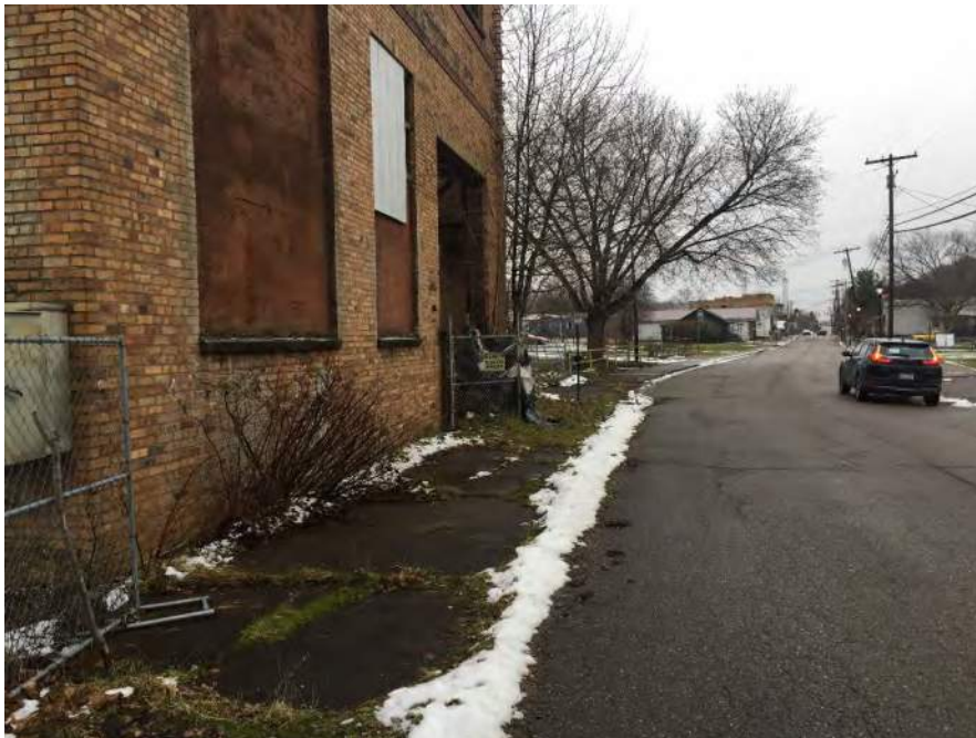
Photograph 16: South Chester Street side of American Industrial Recycling site showing (possible) original concrete sidewalk and potential locations for truck refueling USTs.
