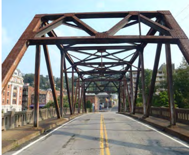
Photograph 2. Steel-decked through Truss of Bridge, with 24-foot Cartway and two 4-foot Sidewalks.
