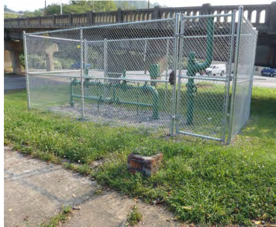
Photograph 10. Gas Regulating Station Located 15 Feet West of the Current Bridge.
