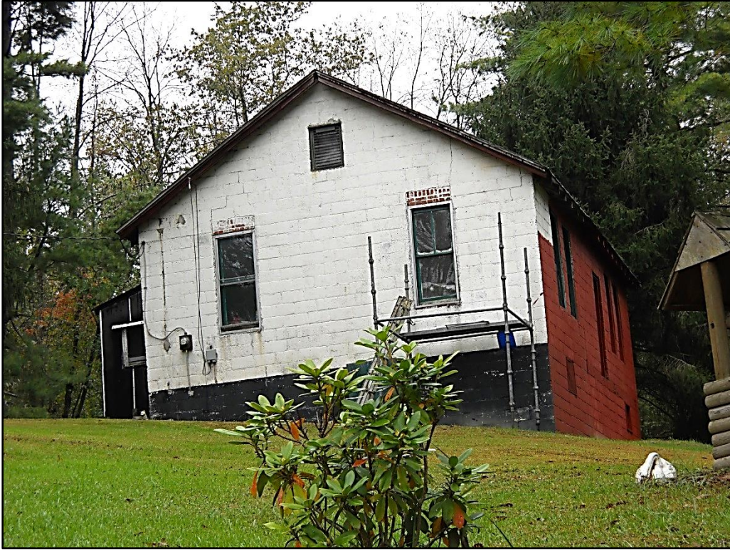
Photograph of AL-1 showing the brick above the windows and the addition, looking east-northeast.
