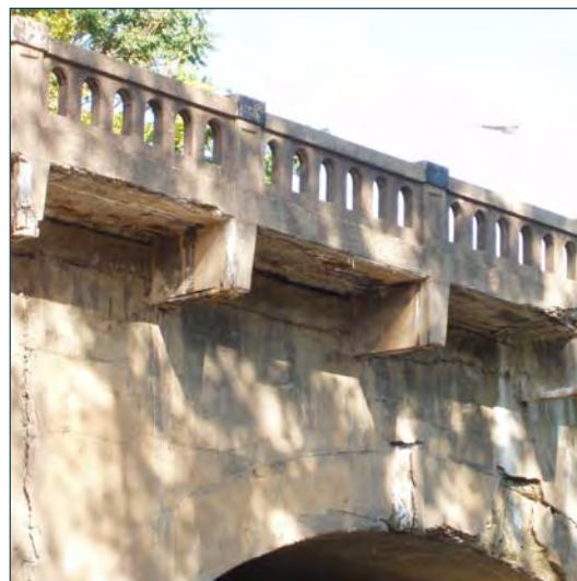
Overhanging Sidewalk Deterioration
