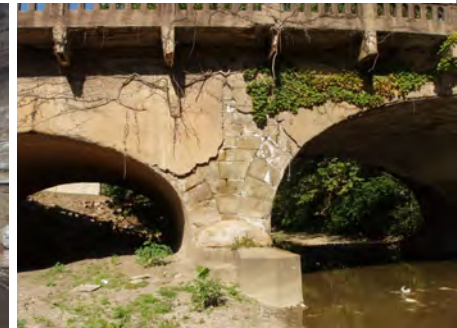
Bridge deterioration prior to veneer removal
