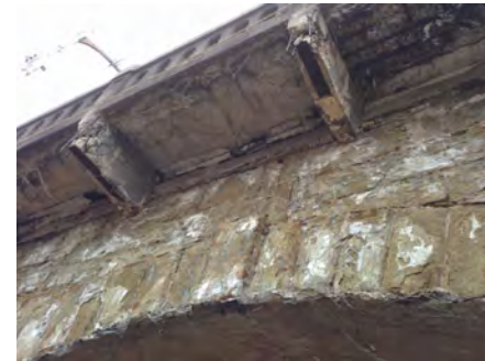
Sidewalk overhang deterioration
