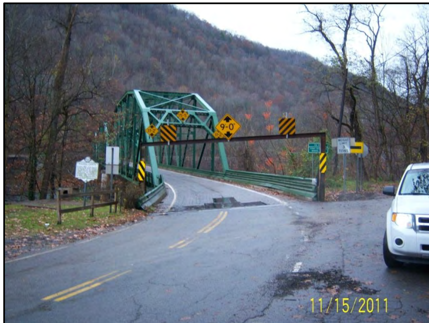
Photograph 1. View of height restricting bar and weight posting at south end of bridge
