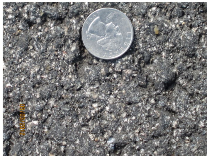
Photo showing close view of raveling from photo above.
